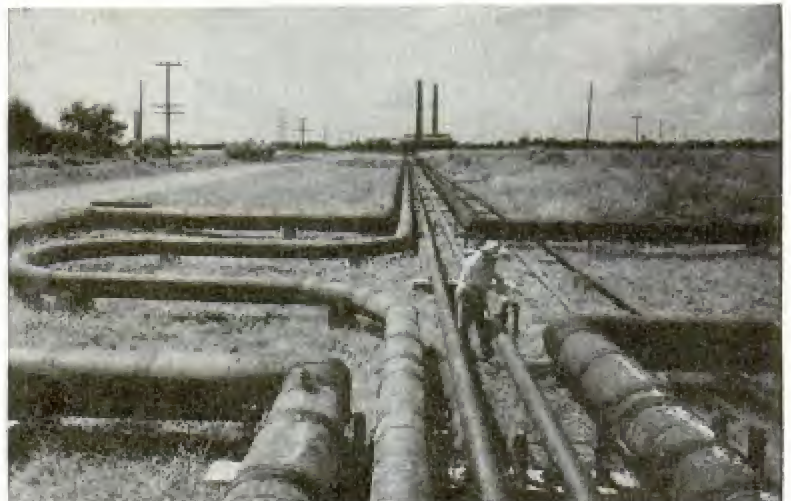
Seventy miles of pipe carry hot water, steam and air into deep sulphur mine in Texas
